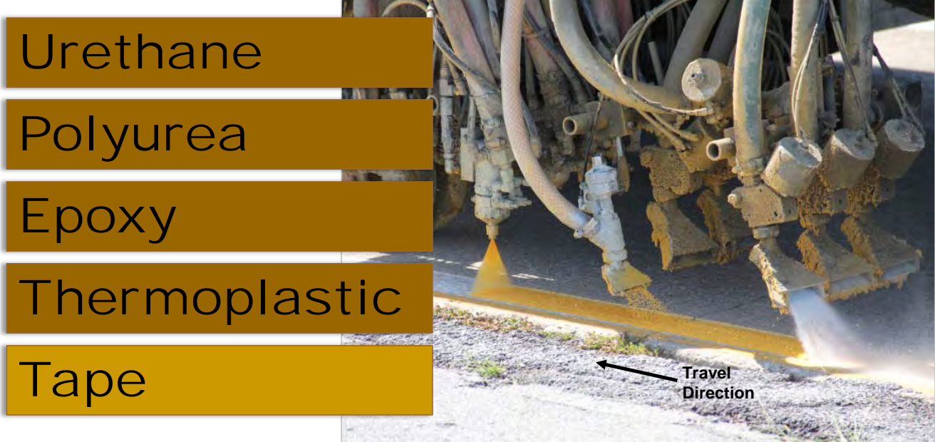
The wet reflective media were delivered to the line prior to the standard IDOT beads, as shown in the photo above. All liquid marking products were placed within a 60 mil groove with the exception of thermoplastic which was installed within a 125 mil groove. The liquid pavement marking products were placed on several types of roadway surfaces (PCC and ACC).
