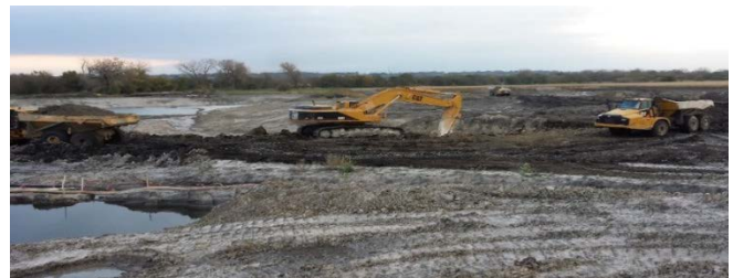
Site-level monitoring of excavator and three haul trucks to evaluate cycle time efficiency
